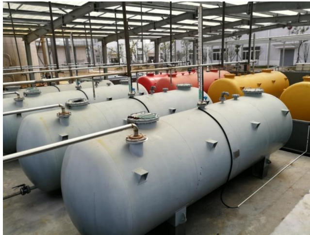
Figure 14. Central business unit Fenton process handling tanks.
