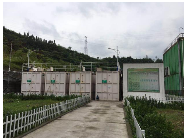
Figure 15. Dazhou Integrated Solid Waste and Wastewater Treatment System.
