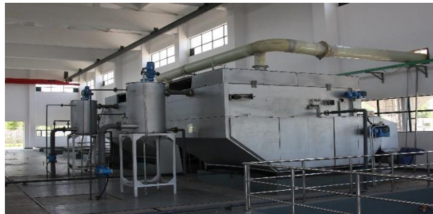
Figure 12. Dewatering facility of one of our North China wastewater treatment plants.
