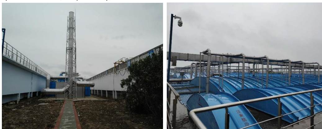
Figure 4. Advanced odour treatment technology incorporated at the Fengxian West Wastewater Treatment Plant of our East China business unit.
