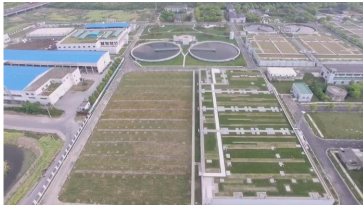
Figure 11. Qingpu Second Wastewater Treatment Plant Phase IV - greenery cover on top of the biological treatment ponds.
