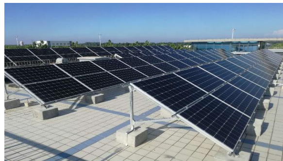
Figure 6. Solar panels installed at the Weifang City Wastewater Treatment Plant of our North China business unit.
