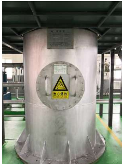
Figure 9. Desulfurization equipment at the Jiamusi City WWTP Sludge Disposal Project.
