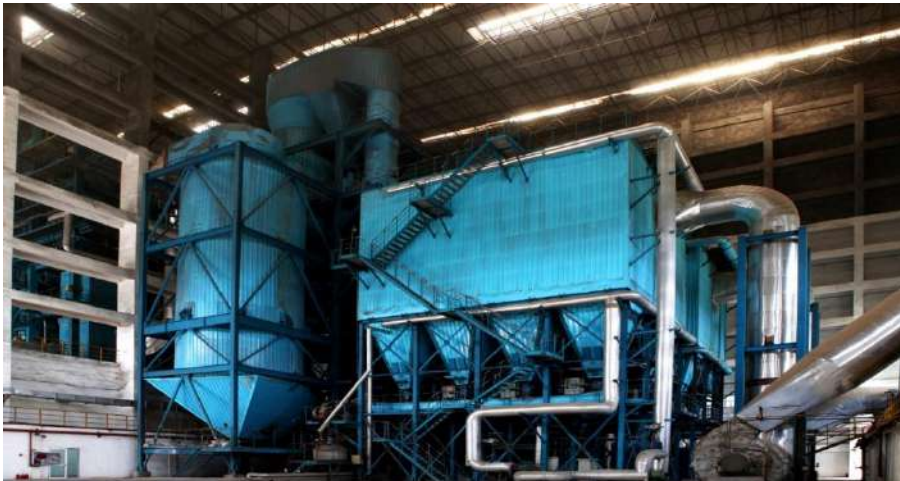
Figure 12. Flue gas treatment system at the Dazhou City Municipal Household Waste Incineration Power Generation Project 1st Phase.
