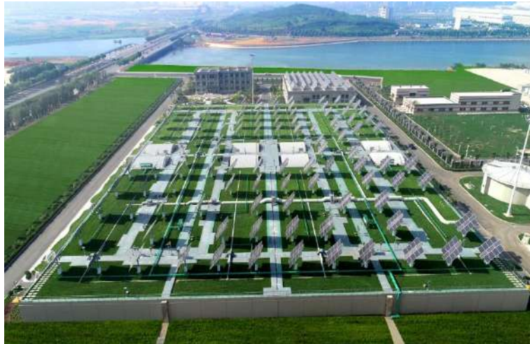
Figure 15. Solar panels installed at the Dalian Quanshui River WWTP Project 2nd Phase.
