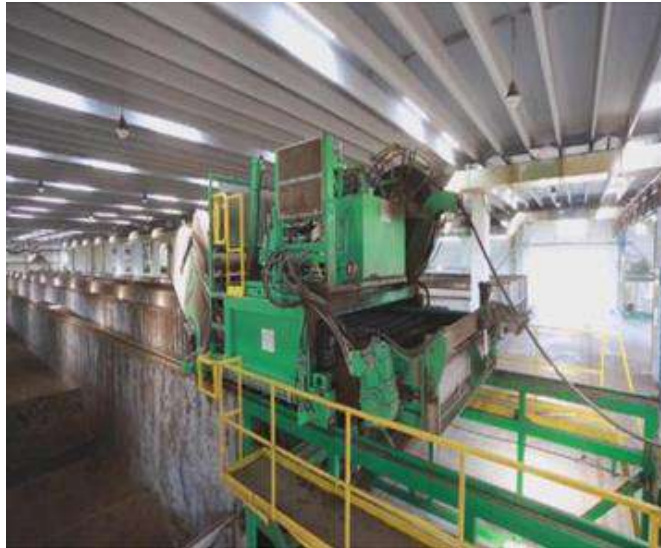
Figure 21. Sludge turner at the Xinxiang City Sludge Treatment and Disposal Project.
