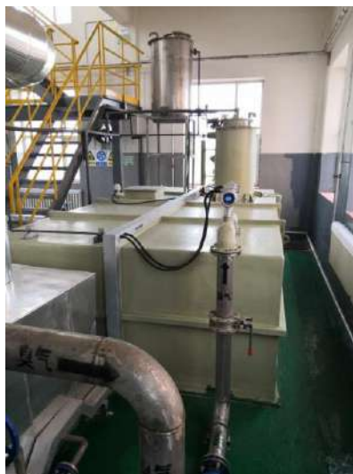
Figure 10. Chemical deodorization equipment at the Jiamusi City WWTP Sludge Disposal Project.
