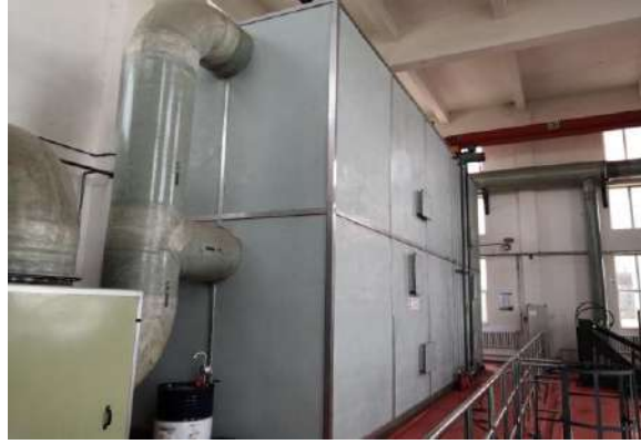
Figure 11. Biological deodorization equipment at the Jiamusi City WWTP Sludge Disposal Project.
