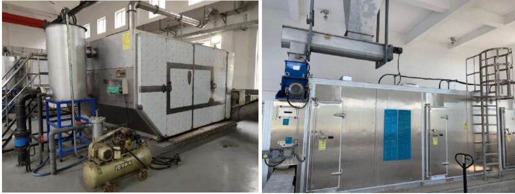
Figure 16. Belt filter press system for sludge dewatering from our North China business unit (left). Sludge desiccation system from our South China business unit (right).
