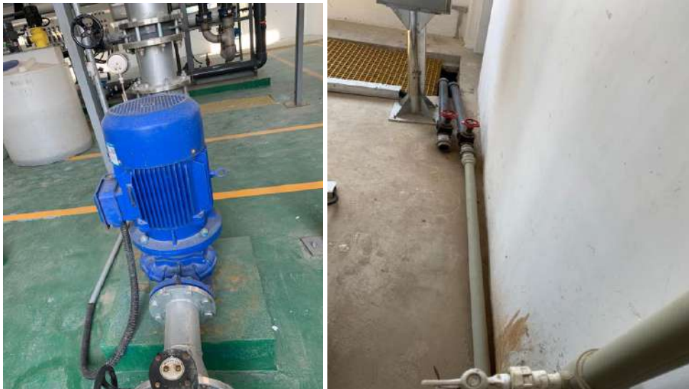
Figure 24. Remodelled pipelines for water recycling at a WWTP from our South China Business unit.
