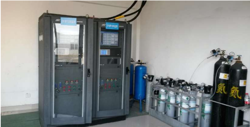
Figure 13. Flue gas online monitoring system at the Dazhou City Municipal Household Waste Incineration Power Generation Project 1st Phase.
