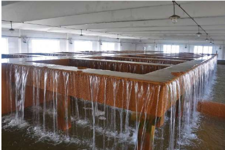
Figure 17. Filter cells at the Jiamusi City Water Supply Project.
