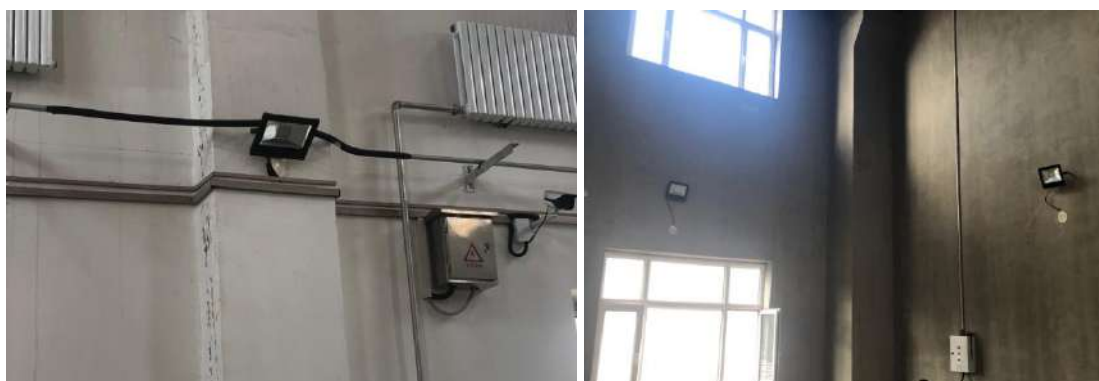
Figure 22. Energy efficiency lighting system at the Mudanjiang City WWTP Sludge Disposal Project.
