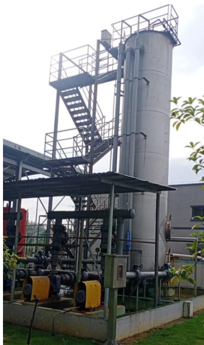
Figure 3 During the Reporting Period, our Yongxin County Industry Development Zone Comprehensive WWTP Project engaged the Fenton treatment system, further increasing COD removal rate.
