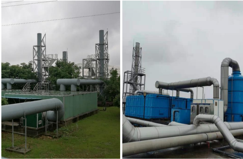
Figure 6 Odour treatment systems at our Hanxi WWTP (left) and Fengxian West WWTP (right).
