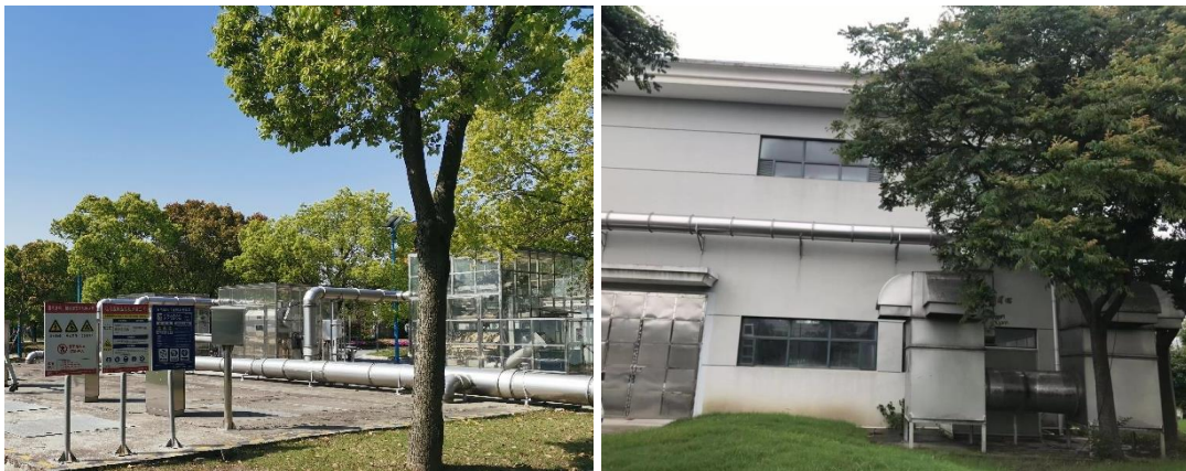
Figure 5 The coarse screening unit, and sludge dewatering unit at Qingpu Second WWTP Project.
