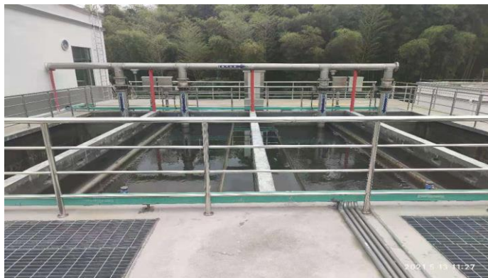
Figure 4 Denitrification deep-bed filtration unit at our Jiangxi Province Yihuang Industrial Park WWTP Project.
