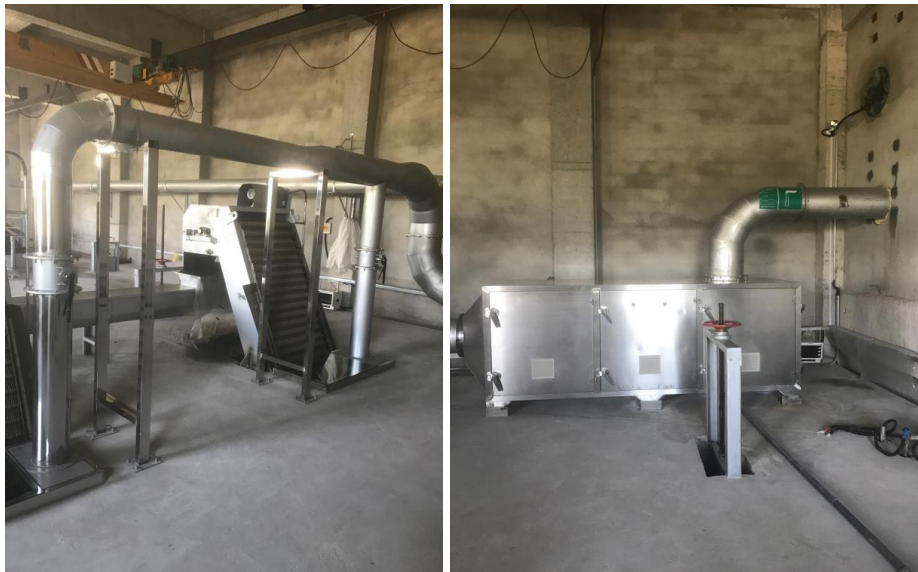
Figure 7 Fine-screen deodorisation facility at our Harbin City Hulan District Old Town Second WWTP Project.
