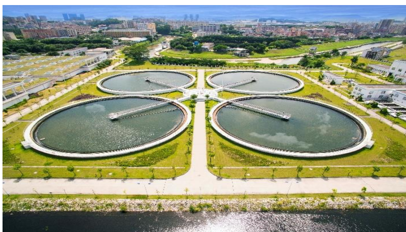
Figure 13: Shenzhen City Guanlan Wastewater Treatment Plant
