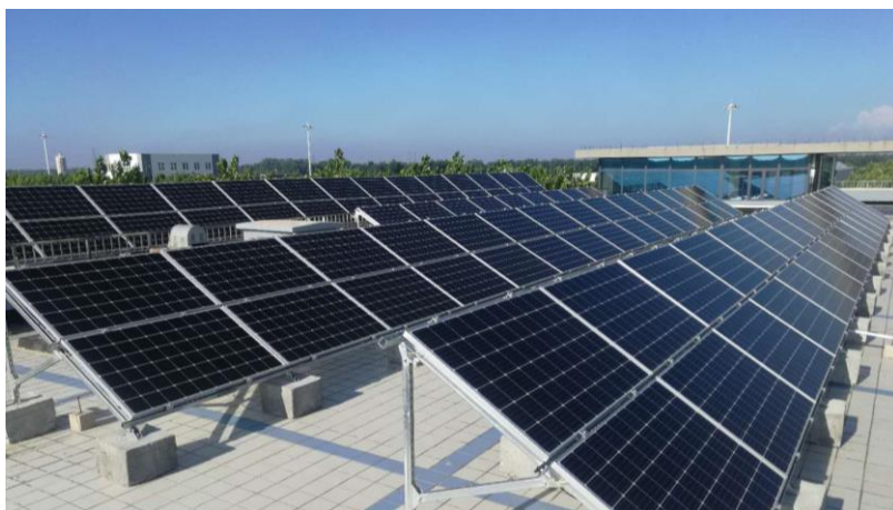
Figure 11: Solar panels installed at one of our North China water supply plants
