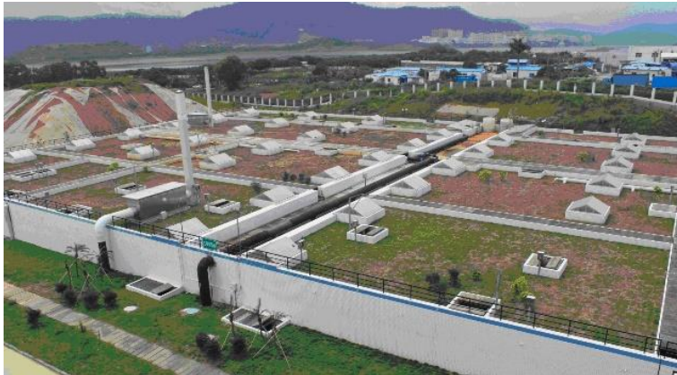
Figure 9: Biological treatment pool at our Shenzhen Egongling Wastewater Treatment Plant
