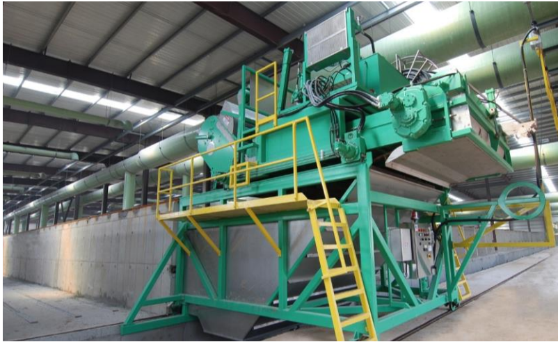
Figure 17: Siemens Bio-fermentation rotary machine
