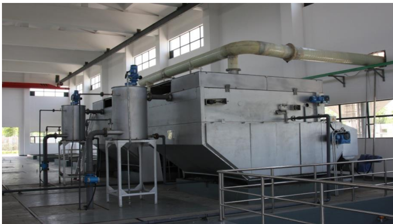
Figure 18: A sludge dewatering facility at our Qingpu Second Wastewater Treatment Plant of North China
