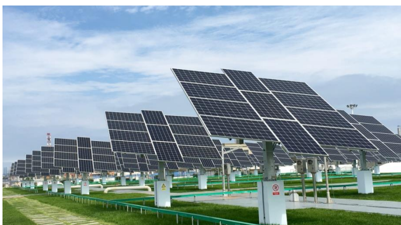
Figure 12: Solar panels installed at our Dalian Quanshui River Wastewater Treatment Plant Project (2 nd Phase)
