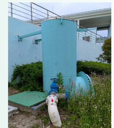
Reclaimed water tank in the water treatment project of North BU
