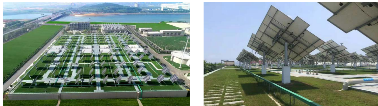
Solar panels installed at the Dalian Quanshui River WWTP Project 2 nd Phase
