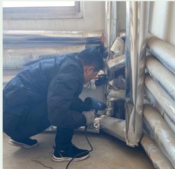
The project company of water supply conducted thawing for pipeline in extremely cold weather
